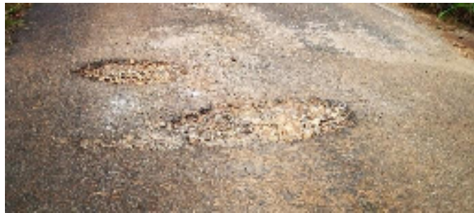
Gambar 2.7 Lubang ( Potholes ) (Sumber : Suwandi, 2018)
