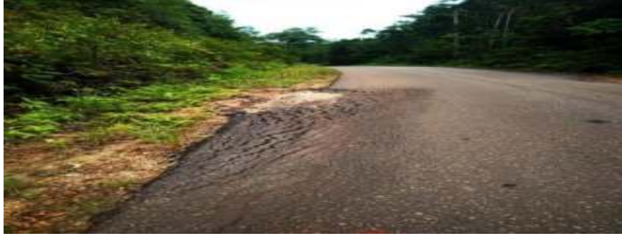
Gambar 2.8 Cacat Tepi Perkerasan ( Edge Cracking )
