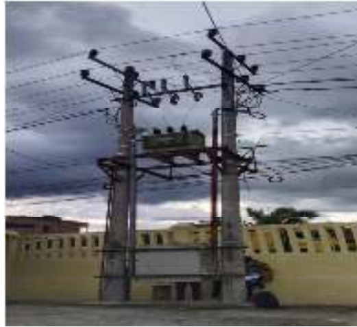
Gambar 2.9. Transformator Distribusi Sb-01
