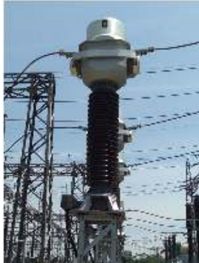
Gambar 3.3 Transformator Arus ( Current Transformers / CT ) G.I TAMORA
