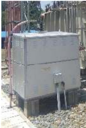
Gambar 3.2 Neutral Grounding Resistance
