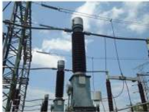
Gambar 3.6 Transformator Tegangan / Potensial Transformer ( PT )
