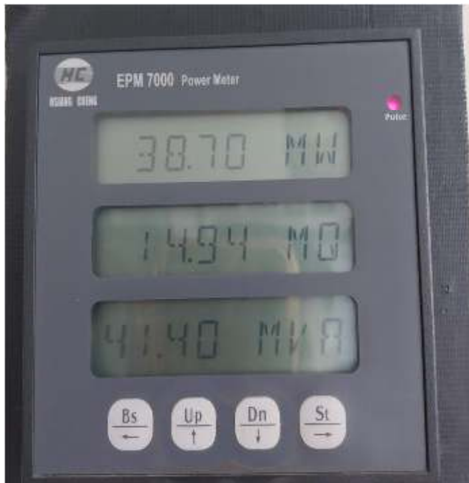
Gambar 3.1 Power Meter Transformator Daya
