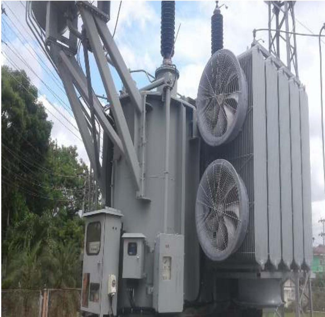
Gambar 3.2 Transformator Daya 3 (TD 3)
