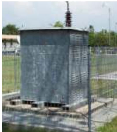
Gambar 2.14 Neutral grounding resistance (NGR)
