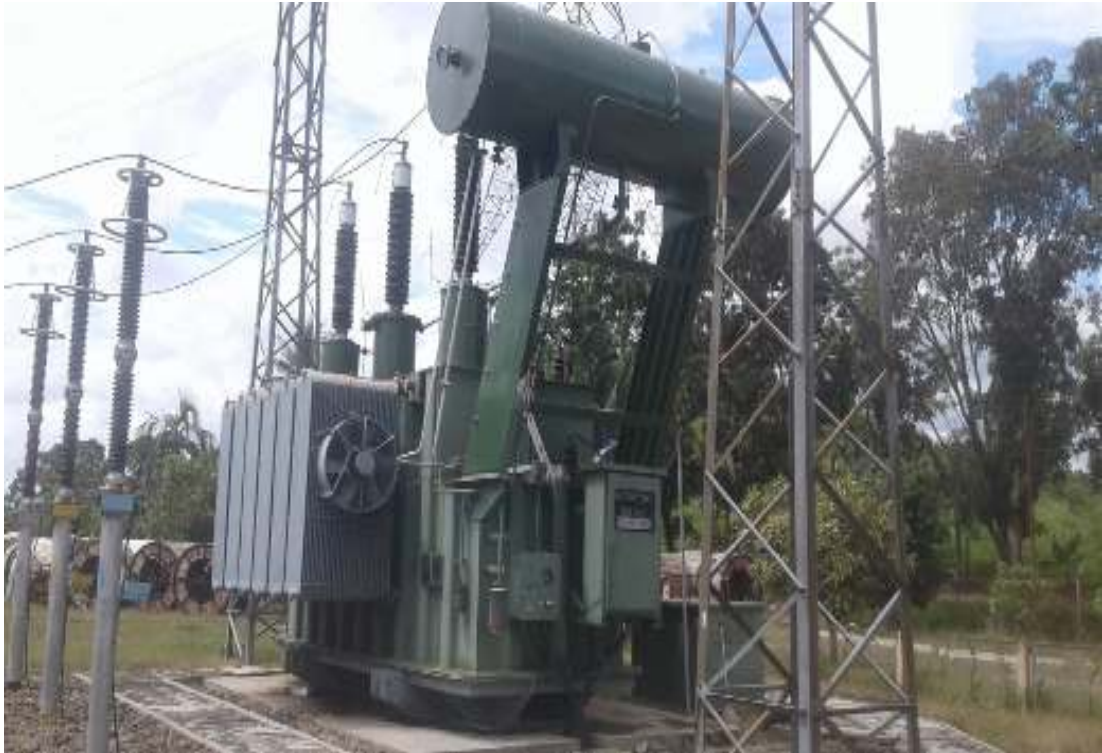
Gambar 3.1 Transformator Daya 2 (TD 2)
