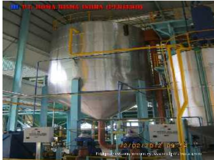
Gambar 3.1 Continuous Settling Tank (CST)
