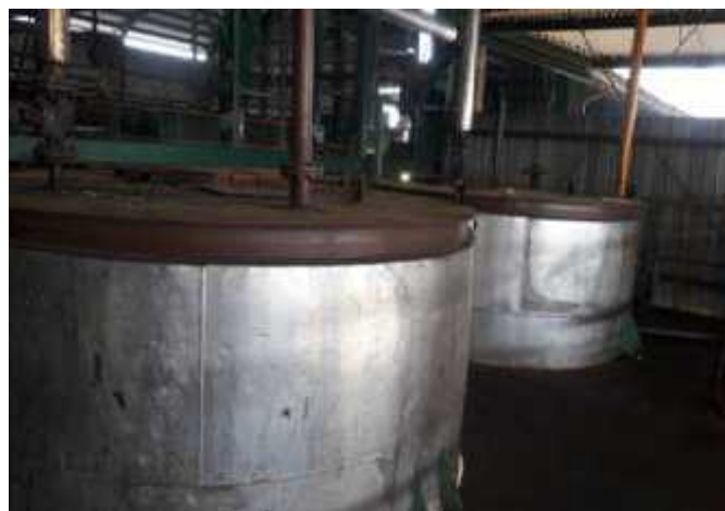
Gambar 3.2 Oil Tank (OT)
