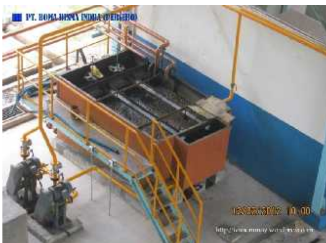
Gambar 4.0 Sludge Drain Tank
