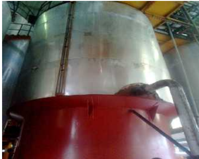
Gambar 3.8 Sludge Buffer Tank
